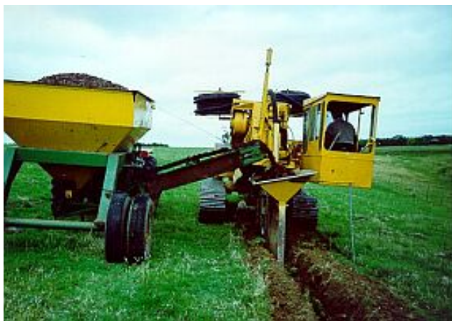
Figure 1. Drainage trencher installing subsurface pipe drains and depositing permeable backfill on top
